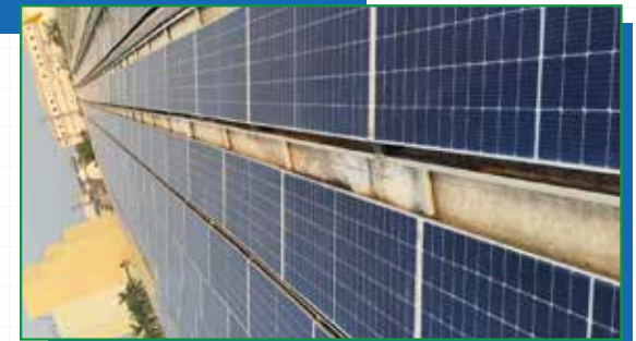
SUBHADRA MALL BARAMATI 390KW
