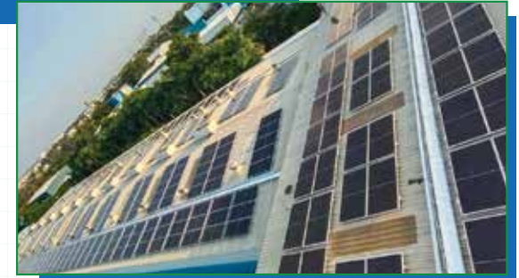
SUYASH AUTO 565KW AT BARAMATI
